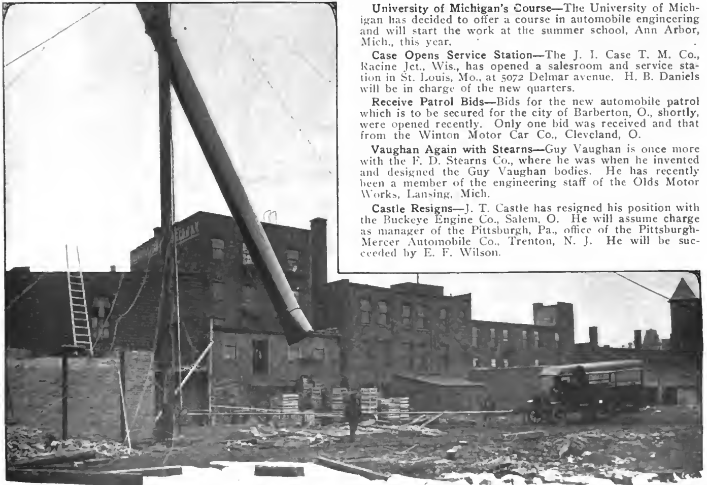
Showing one of the many duties to which a motor truck may be subjected. A White 3-ton truck utilized to hoist an 80-foot sheet-iron smoke stack into its cradle, 12 feet above the ground
